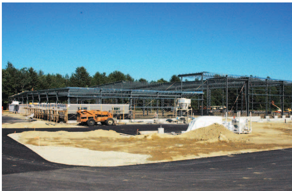
F.W. Webb's pre-engineered Butler building under construction in Dover, N.H. Note the two roof elevations and self-serve entry canopy at the front entrance on the far left.
